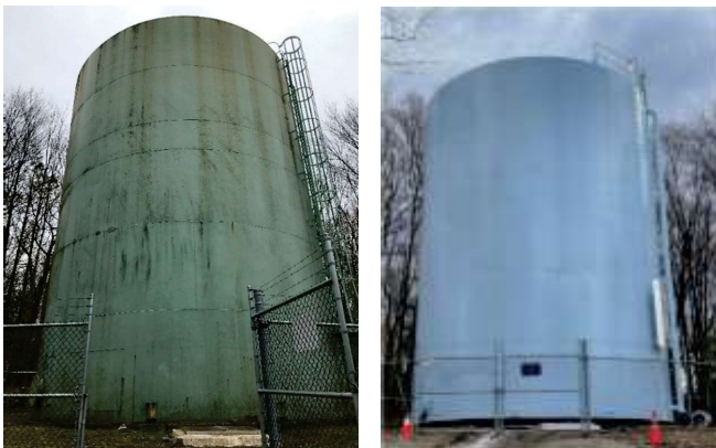
*Photo caption: Before and after photos of a water tank refurbishment in West Milford, NJ.
